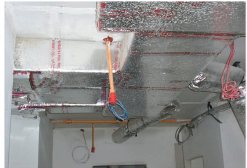
Keep HVAC Ducts sealed during construction
