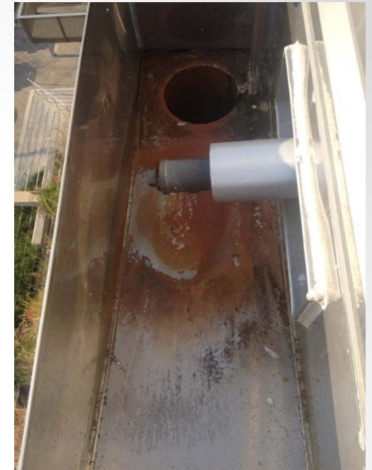
Roof Drain (Rainwater & Cond.)
